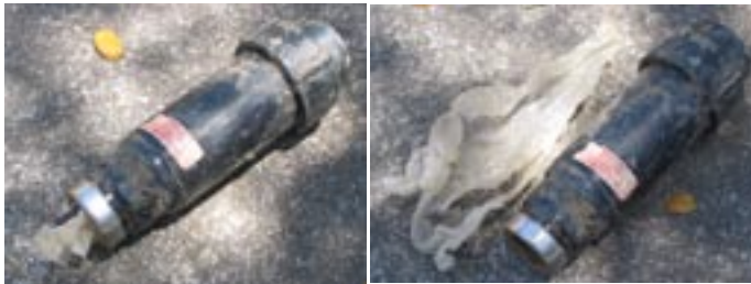
Five major sprinkler heads in the tot-lot area were found to have plastic stuffed inside. To control flow? Now replaced.
