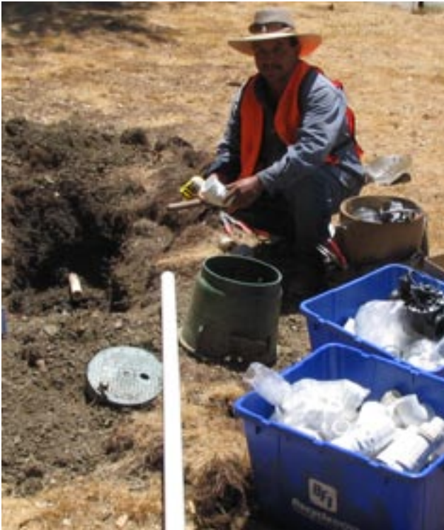
Rogelio Magaña working on the water line repair. Parts readily available in all sizes and shapes.
